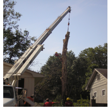
Removal of a Sycamore tree in a back yard with a crane & one of our tree climbers. A job not for the untrained.
